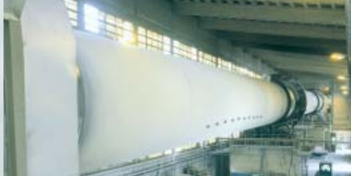
At Pargas, Finland, quick lime is produced by burning limestone in a rotating kiln.
