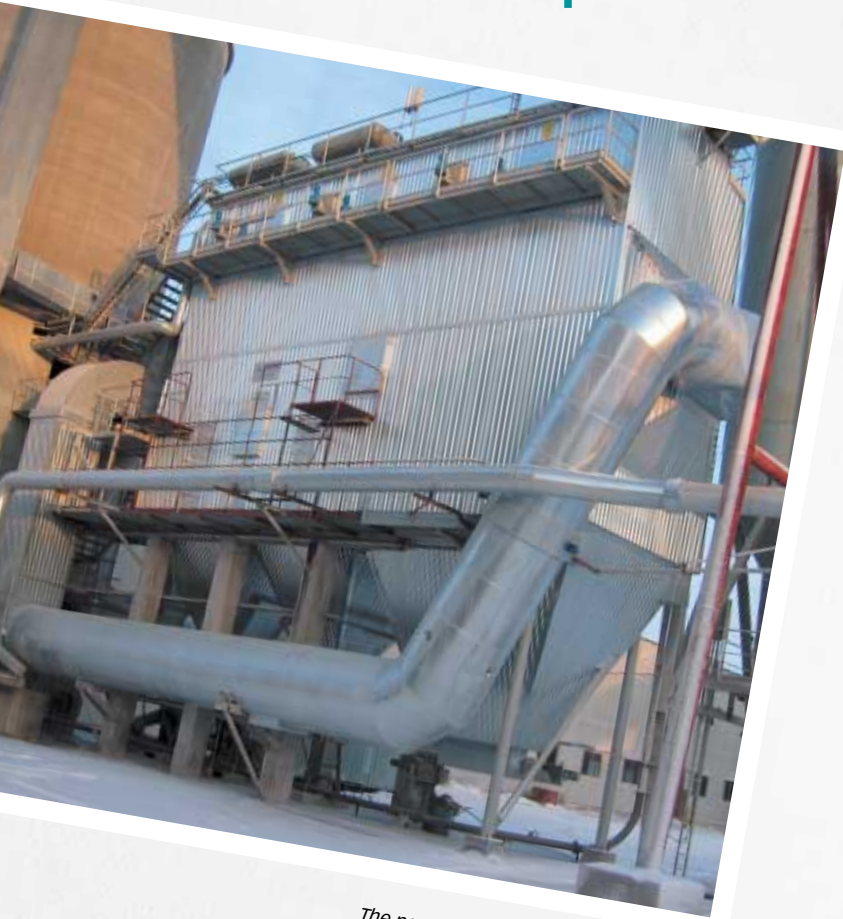
The new filter at the Louhi plant in Finland reduces dust emissions in an effective way.
